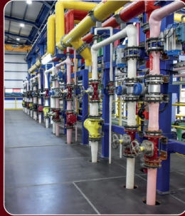
DEIONISED WATER TREATMENT
